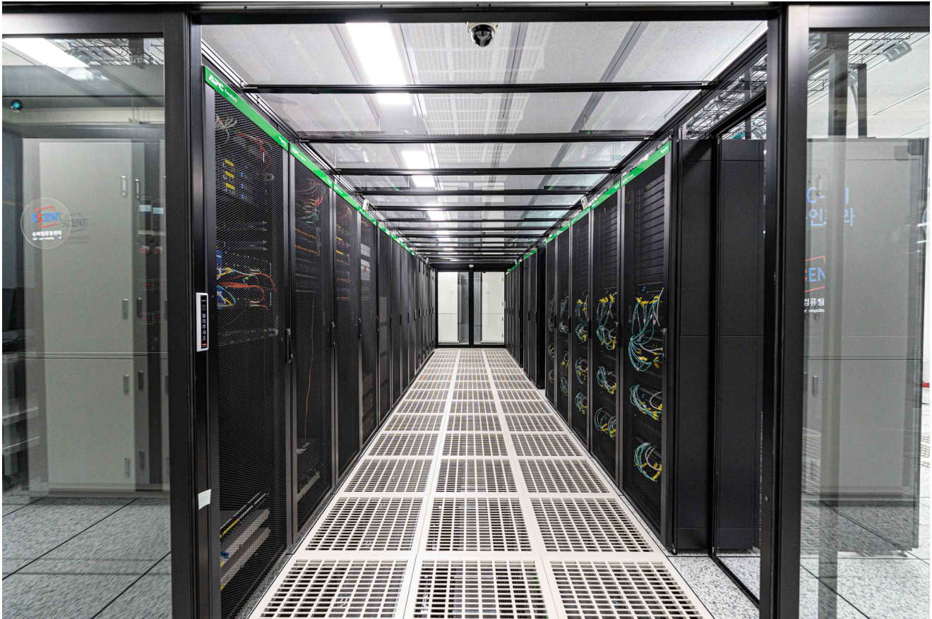
▲ 'HPC-AI public infrastructure cluster' built at GIST AI Graduate School (Super Computing Center)
